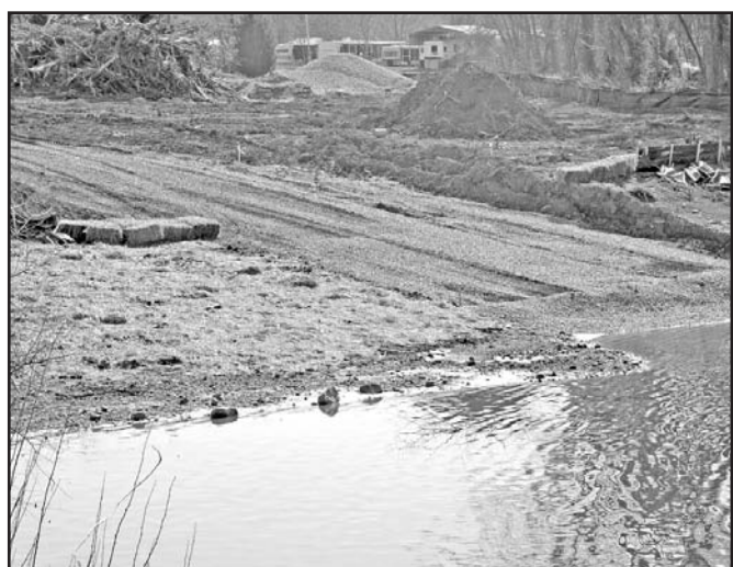
DNR has been busy grading and preparing this area of Hiwassee Mayor's Park for the incoming boat launch and boat dock. Stancil has worked extensively with Mayor Barbara Mathis to make her dream of a Mayor's Park come true.
